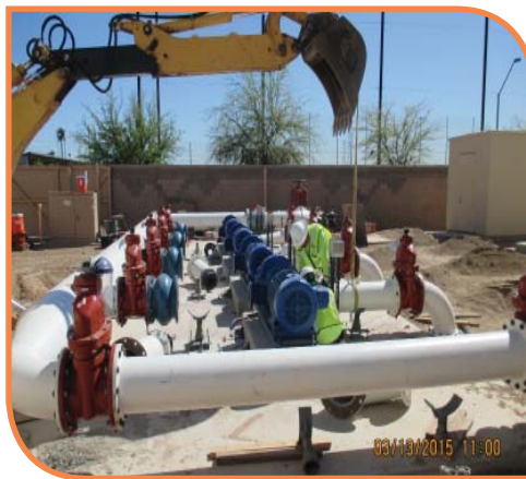
Avondale Northside Booster Station
